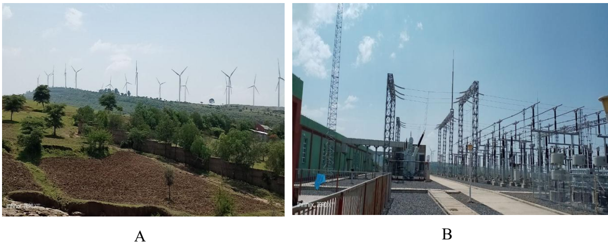
Figure 13 Adama wind farm wind turbines (a) and substation (b)
