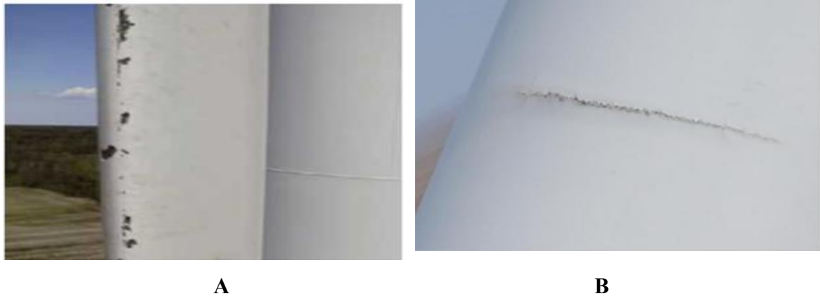
Figure 3: A) The leading edge corrosion [18] and B) Micro cracking [25]
