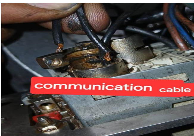
Burnt communication cable Adama wind Farm I
