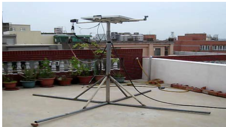
Figure 2.37: Tracking Solar Panel Mount
