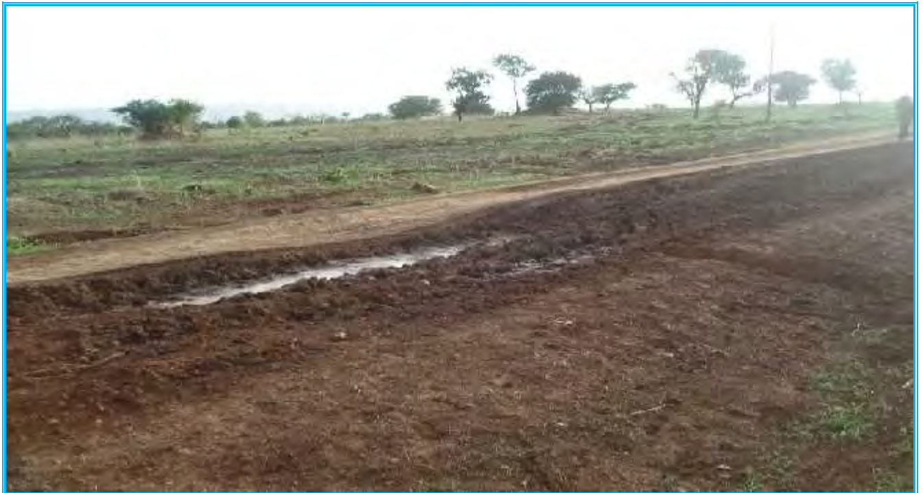
Figure 5.6: Weakened Carriageways at Station 15+500
