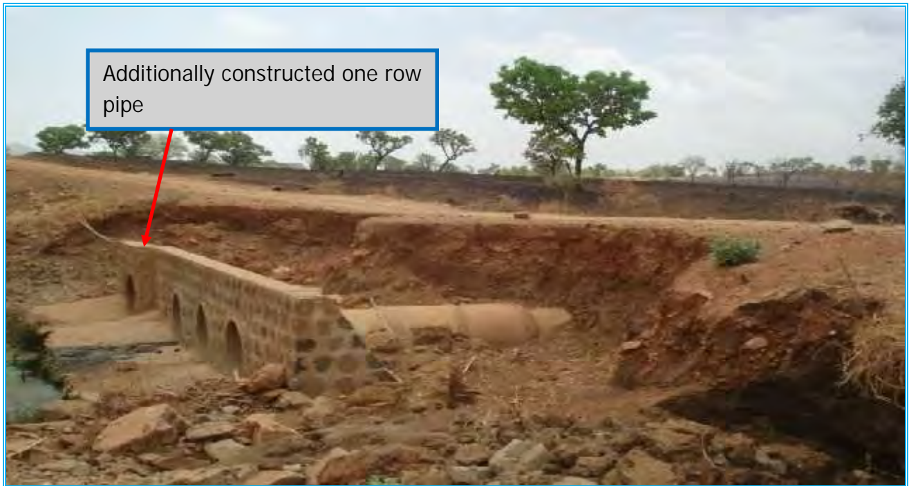
Figure 5.2: Four Rows of Pipe Culvert after one Row Pipe on the left added.
