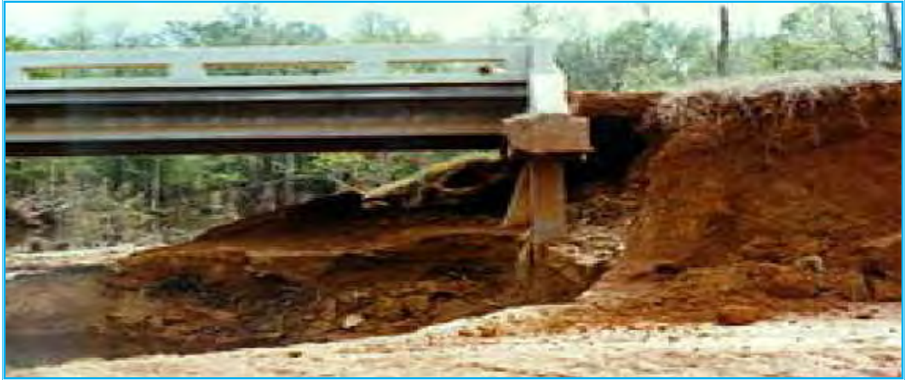
Figure 2.1 Typical Scour of Bridge at Abutment
