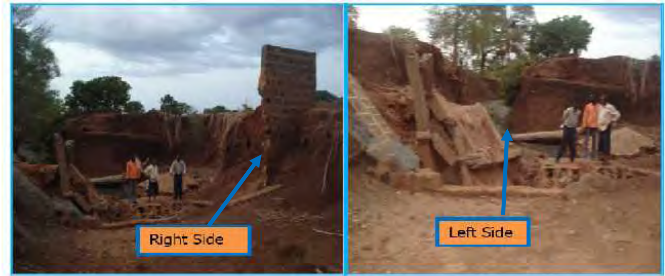
Figure 5.5: Damaged Slab Culvert at Station 41+700
