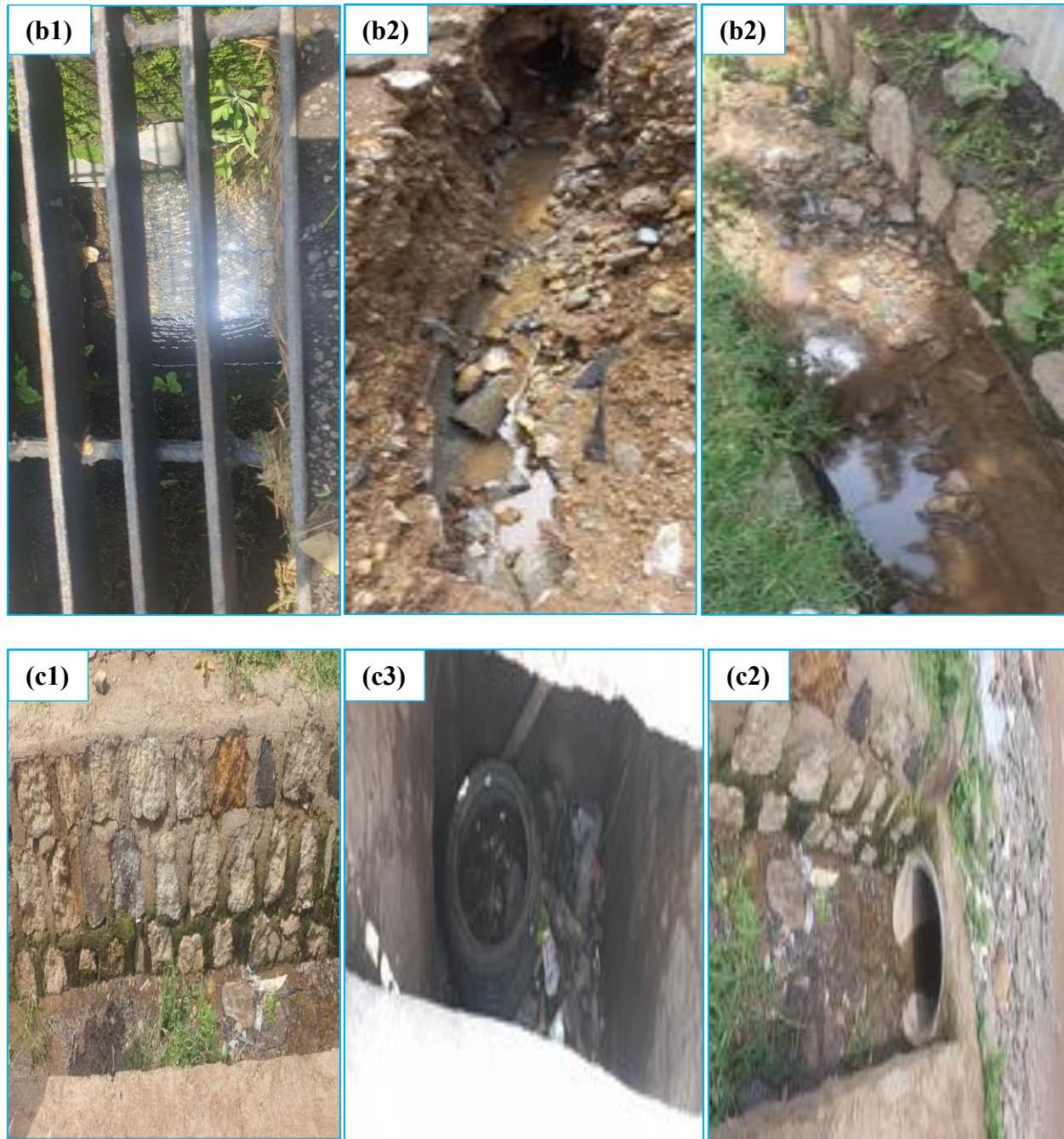
Appendix Figure 1: Photographic examples of “Good,” “Fair,” and “Poor” conditions for key performance criteria. (a) Structural integrity ( C_2 ): a1 = Good (intact concrete, no cracks), a2 = Fair (minor cracking), a3 = Poor (severe cracking, spalling). (b) Erosion control effectiveness ( C_3 ): b1 = Good (well-vegetated, stable banks), b2 = Fair (minor scouring), b3 = Poor (severe gully, bank failure). (c) Sediment accumulation ( C_4 ): c1 = Good (<25% blockage), c2 = Fair (25-50% blockage), c3 = Poor (>50% blockage).
