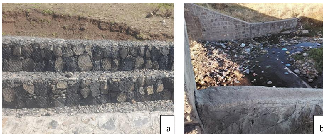
Figure 4:33 Flood control and protection mechanisms implemented in Debre Birhan city: meshed gravel gabion (a) and masonry retaining wall (b). Source: computed by the author (2023).
