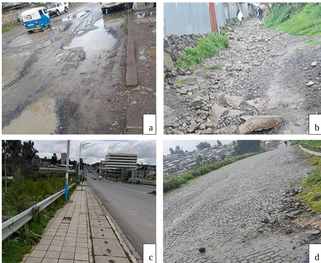
Figure 4:15 Existing road types and conditions in Debre Birhan city: surface deteriorated asphalt road (a), surface deteriorated gravel road (b), asphalt roads and walkway (c) and cobblestone road (d). Source: author's computation (2023).
