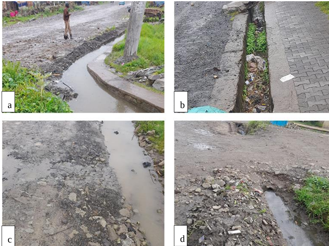
Figure 4:13 Drainage systems in Debre Birhan city: open drainage caused flooding (a), open drainage filled solid waste (b), open drainage creating land pollution (c) and closed drainage line (d). Source: author (2023)
