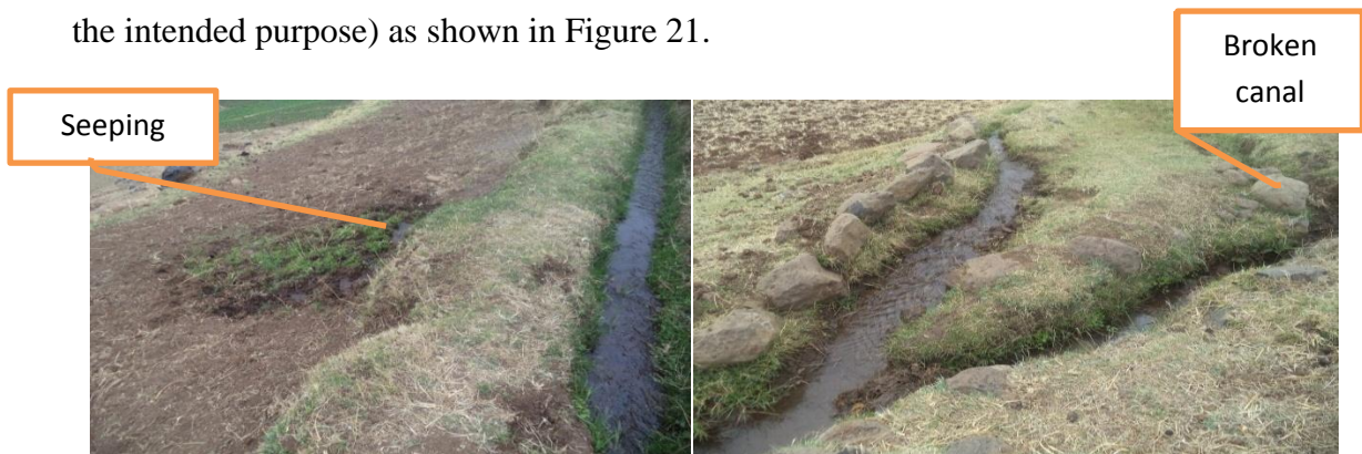
Figure.20 Photos showing canal problem
