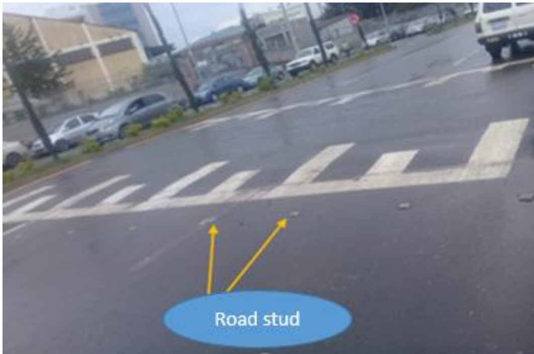
Figure 4- 22 Photo shows reflectors on hump
