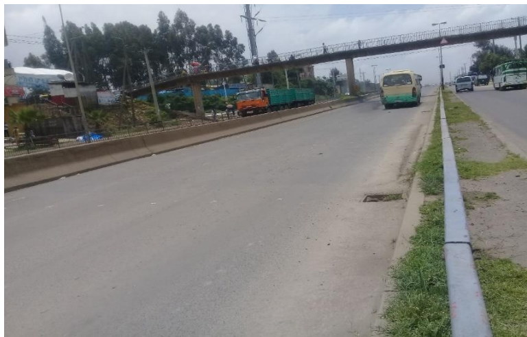
Figure 4- 12 photo show not road marking
