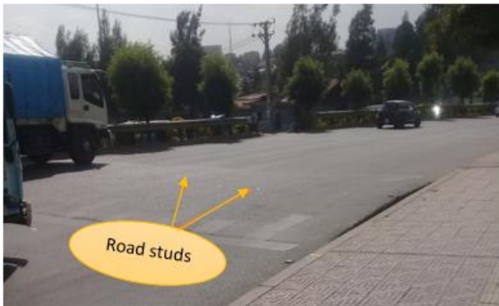
Figure 4- 3 Reflectors on hump
