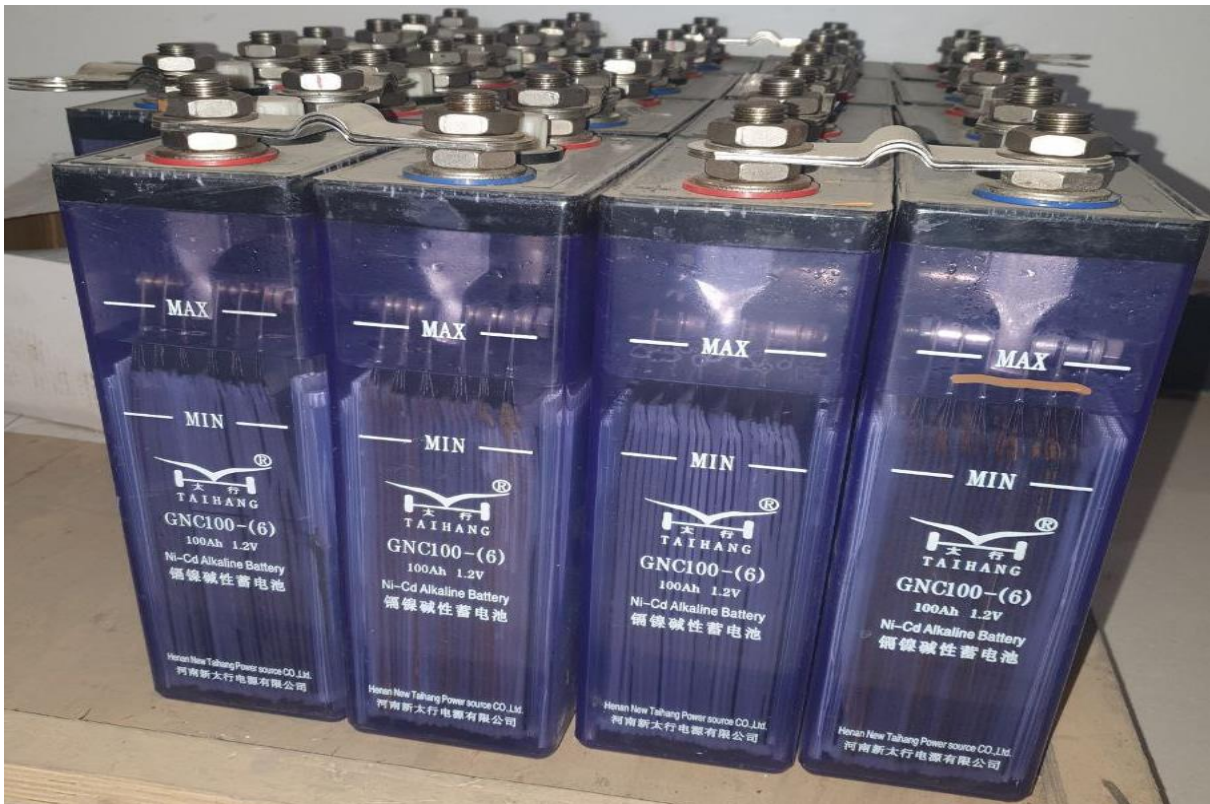
Figure 3. 6: Ni_Cd Alkaline Battery Set at AALRT (in maintenance room)
