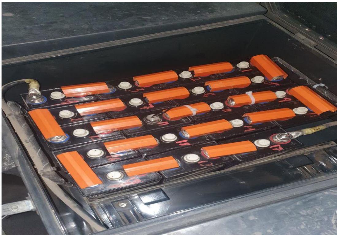
Figure 3. 5: One Installed Battery Set of 19 Individual Batteries.
