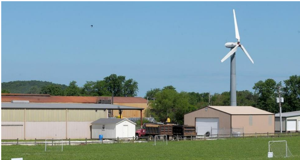
Figure 2.4 Wind turbine for an industry in Arkansas, USA [31]
