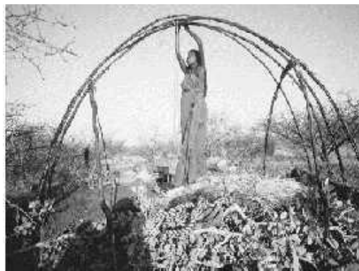
Photo .2.2 a Somali traditional house that has been on starting of construction ( http://shafisaid.wordpress.com/tag/Somali-nomads/ )
