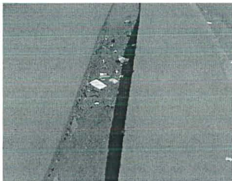
Figure 4.6 Picture showing Un maintained roads
