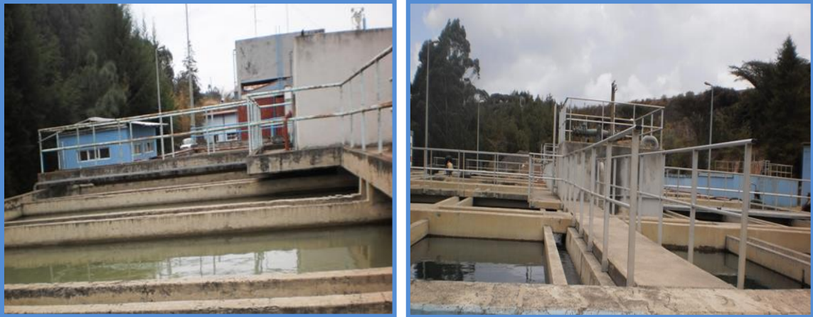
Stage one and stage two-pulsator type Clarifier
