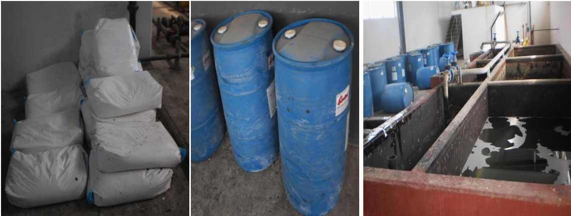
Chemical dilution and dosing
