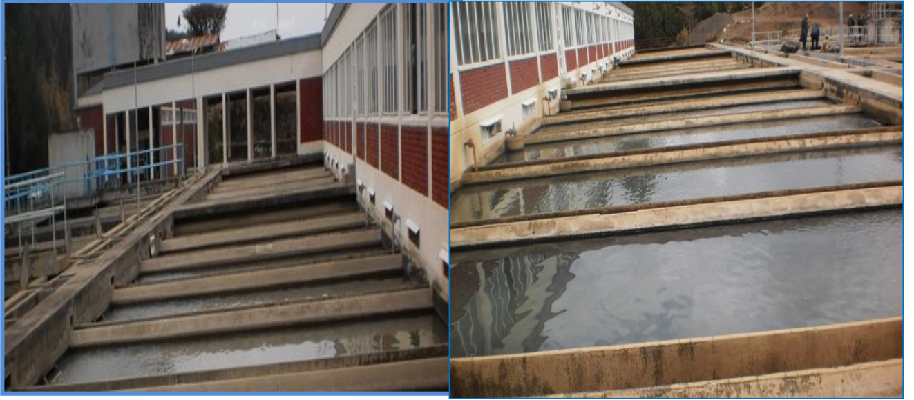
Stage one and stage two rapid sand filter bed
