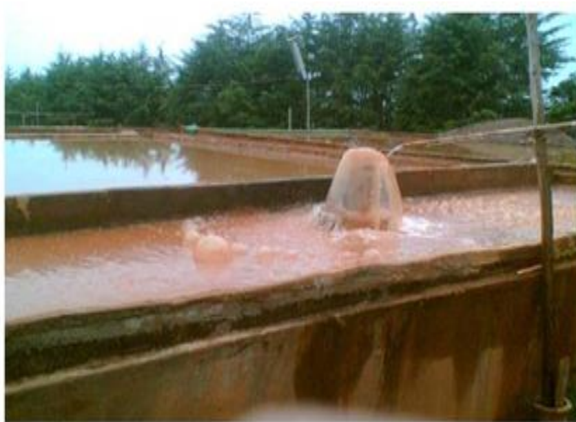
Figure 3-4: The primary sedimentation tank at treatment plant when Aluminum Sulfate added
