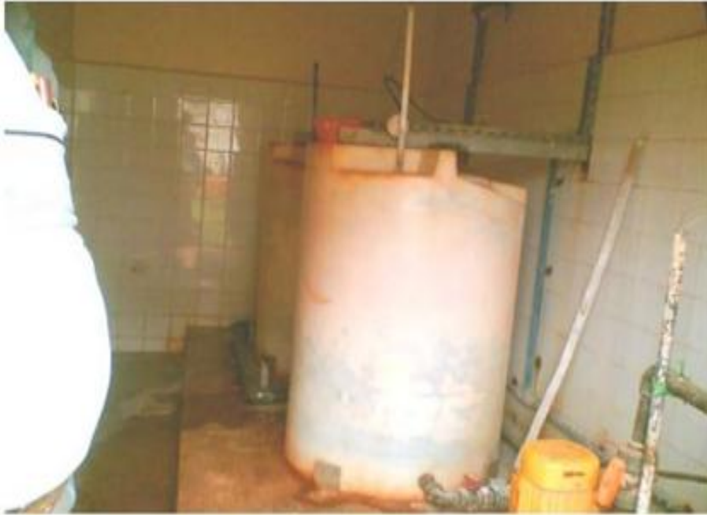
Figure 3-5: Mixing systems of chlorination at clear water tank
