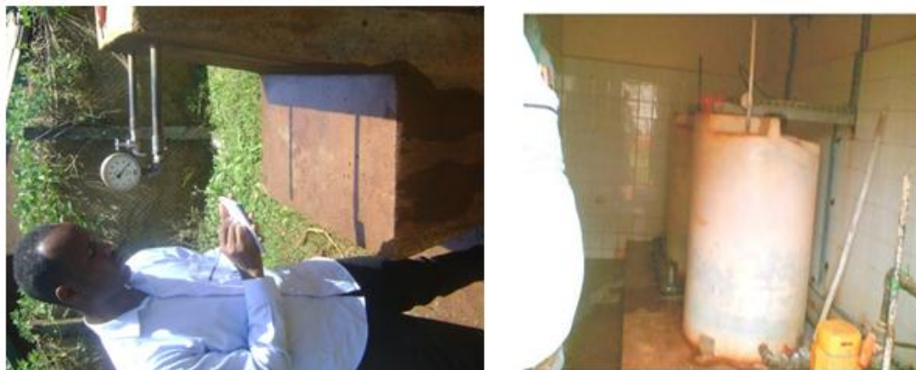
Figure 3-9: Pressure and residual chlorine field measurement
