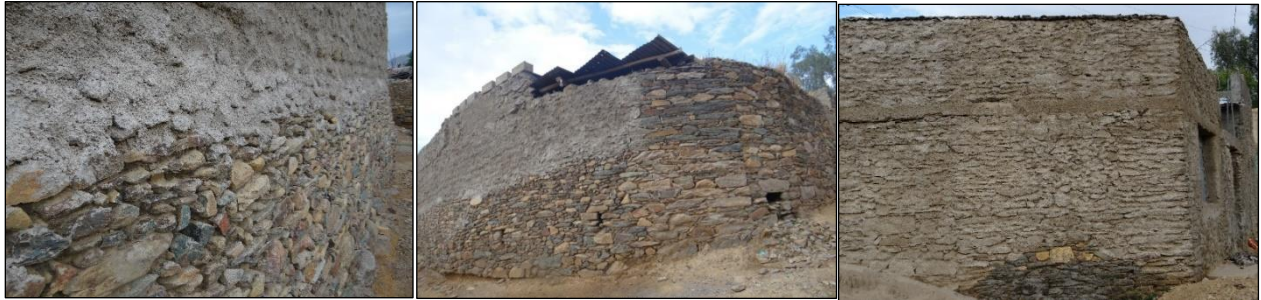
Figure 130: Incompatible Maintenance and Restoration and renovation of historic Buildings.
