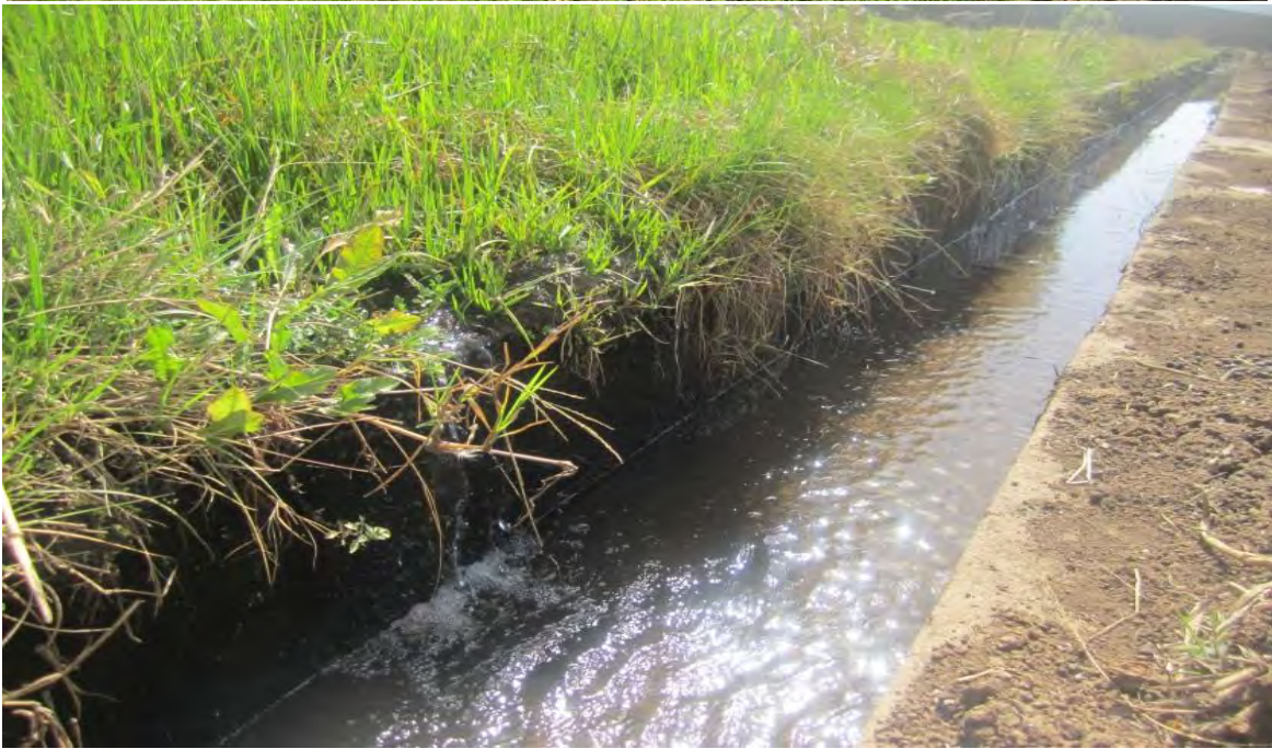
Photo-2 Seepage water from the foot of spillway side wall entering to outlet
