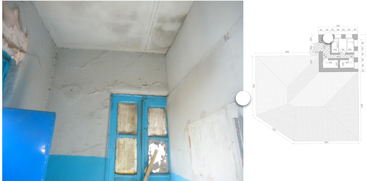
Figure 34: Plaster detachments showed at the wall and rainwater seepage showed at the ceiling
