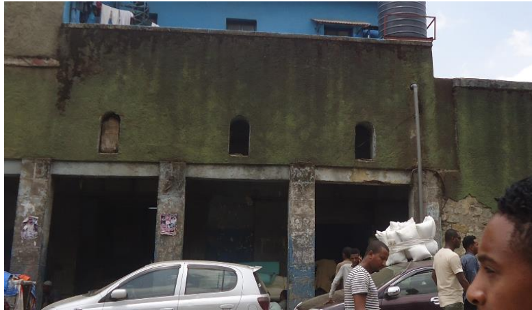
Figure 36: Discolorations and dilapidation exhibited on the NW view
