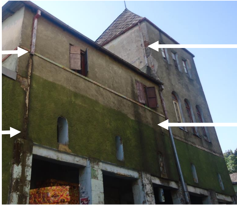
Figure 38: Discoloration and plaster detachments happened because of the malfunctioning of the drainage system exhibited on the NE view
