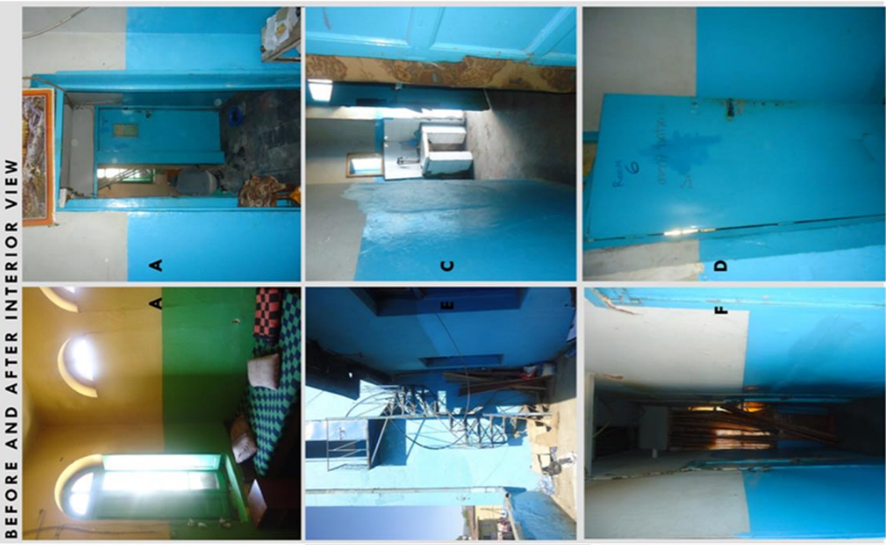
Existing conditions of the different angles and spaces of the building interior: before the proposal
