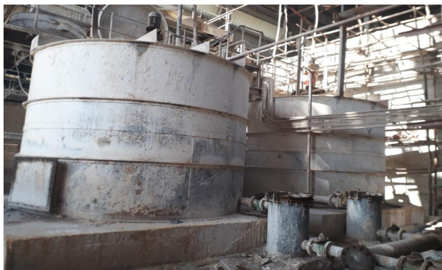
Figure 2. 5: The WSSF milk of lime preparation plant
