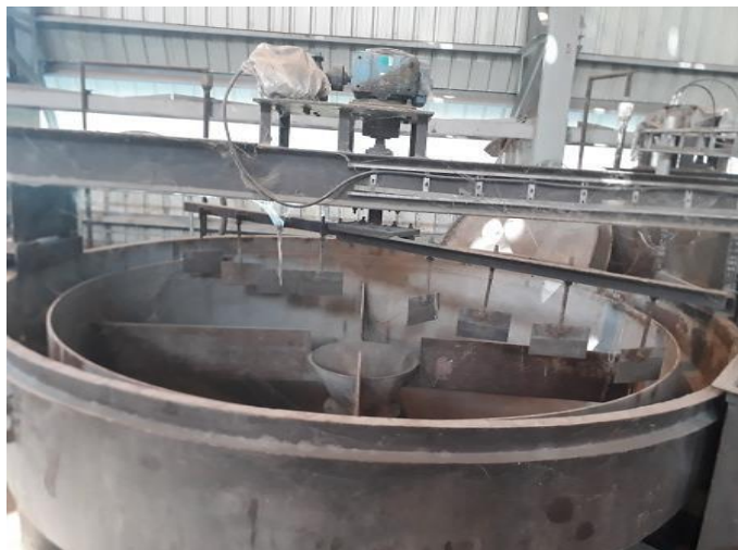
6. 1: Photo of flotation filtrate juice clarification plant
