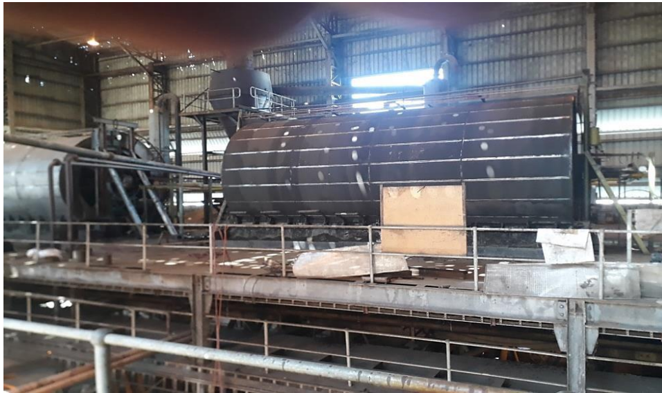
Figure 2. 4: WSSF Rotary Vacuum Filtration Plant
