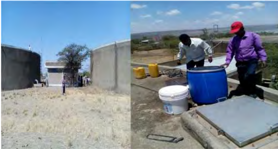
Figure 4-2: Constant Head Drip chlorination on top of 2000m 3 and 4000m 3 reservoirs
