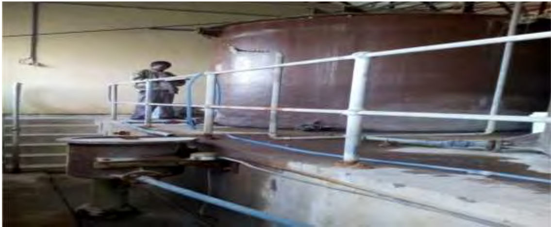
Figure3-14: Mixing and dosing systems of chlorination to Treatment plant (USB Rapid Sand clarifiers)
