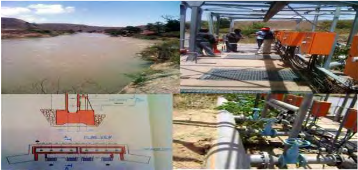
Figure3-10: Adama Water Supply Concrete River Side Box intake and row Water Pumping Station
