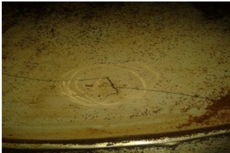
Figure 5-13: Shows the initial crack due to manufacturing and the propagation of new due to operation.
