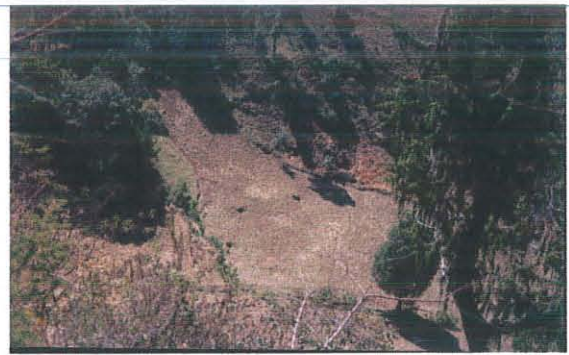
Figure 7.2 Landslide scar that damage property
