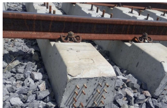
Track super structure material
