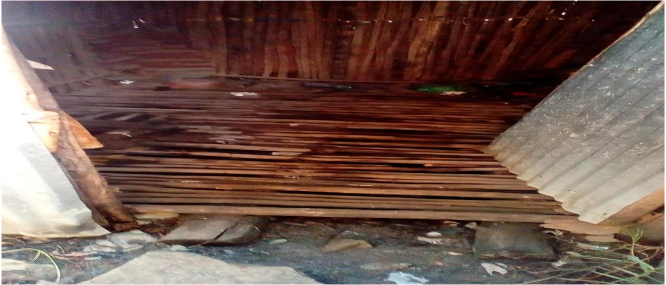
Already filled toilet but used by 20 people or 5 HH. (Latitude = 8.97690, Longitude= 38.74568)
