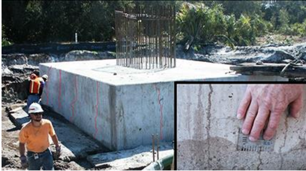
Figure 1.1 Early Age Thermal Cracking on a Massive Foundation ( https://www.concretebridgeviews.com )
