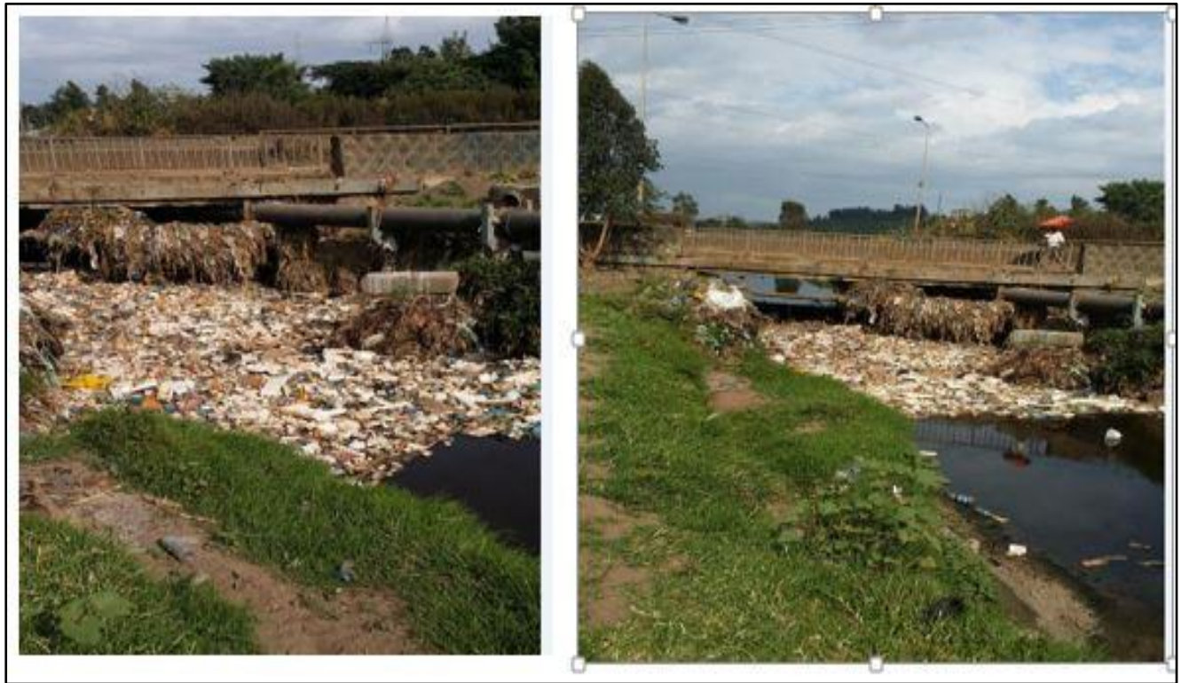
Figure 1 Trash accumulation and blockage of the bridge
