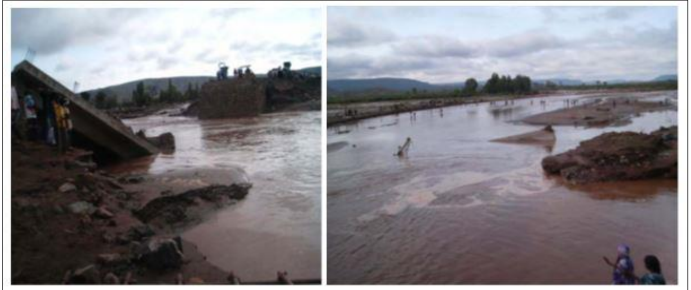
Figure 5 Fail Fafem River Bridges and Fafem River Flooding Condition.
