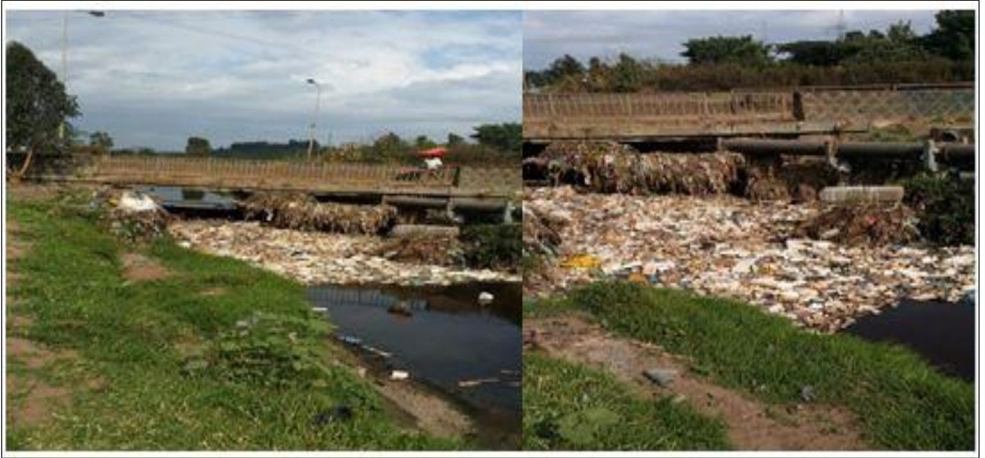
Figure 7 Accumulated Trash on inlet of Bridge
