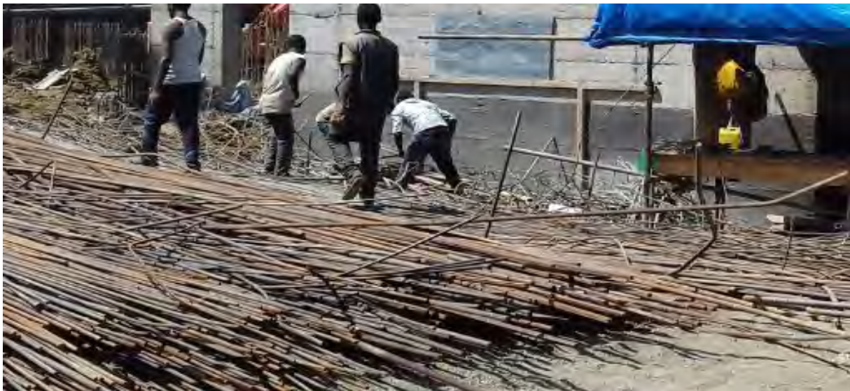
Fig 4.5: stacking of different sizes of reinforcement bars and the damaged reinforcement bars
