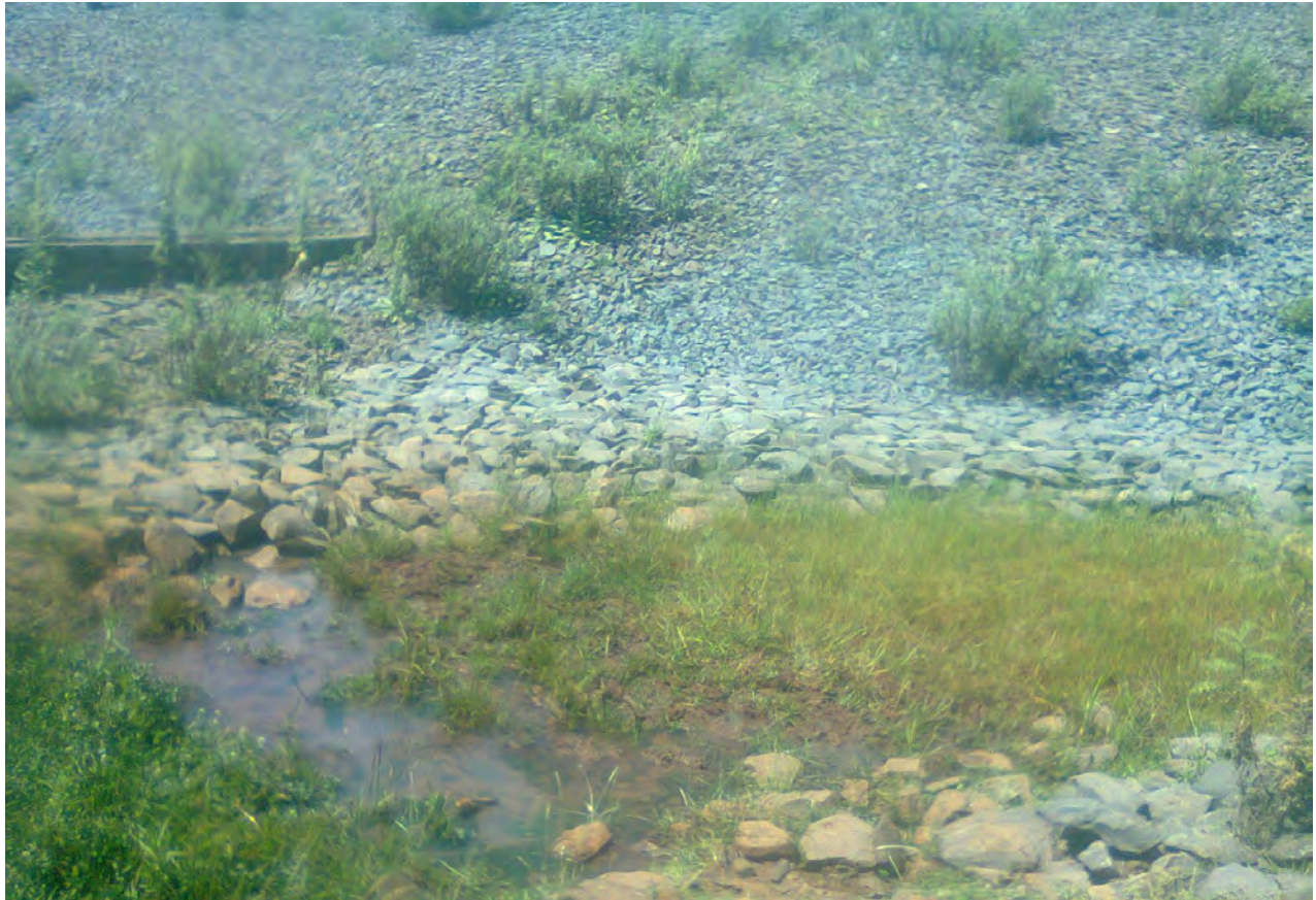
Fig 1.5: Seepage areas at downstream berm.
