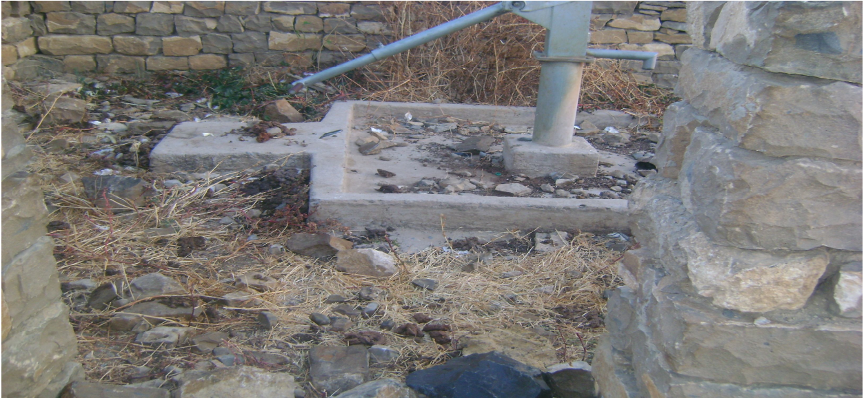
Figure 3.2: The damaged hand pump which used as a toilet by the local community.
