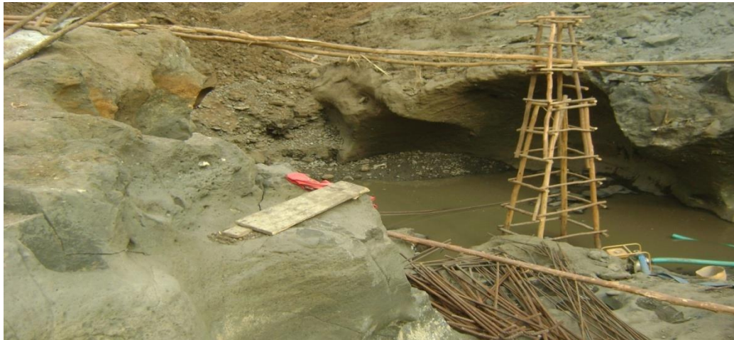
Photo 4: Cavity encountered at the center of the weir axis during foundation excavation
