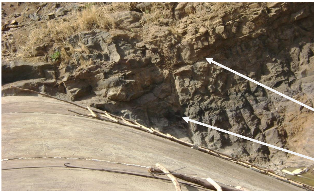
Photo 5: Left abutment d/s of the weir, one vertical joint intersecting in to the structure foundation and one horizontal joint
