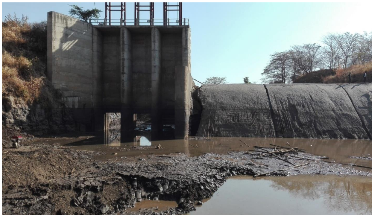
Photo 2: Tana Beles diversion head work (Dec 2017)
