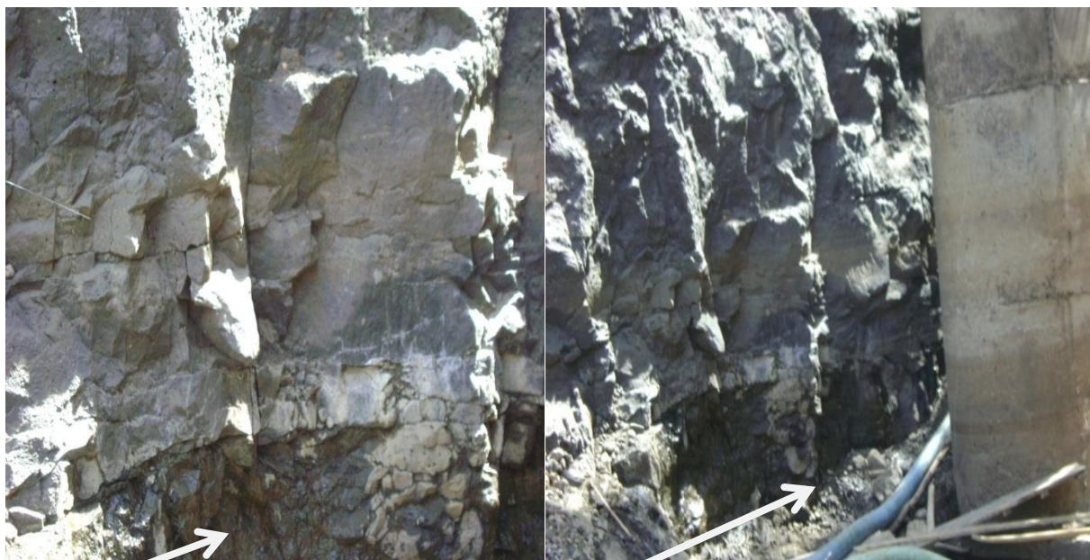
Photo 7: Seepage through sheared rock at right abutment at the side of the under sluice structure
