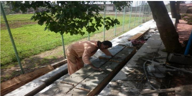
Figure 3.5: Beam Casting Sample (From Adiss Ababa University Institute of Technology Civil Lab)
