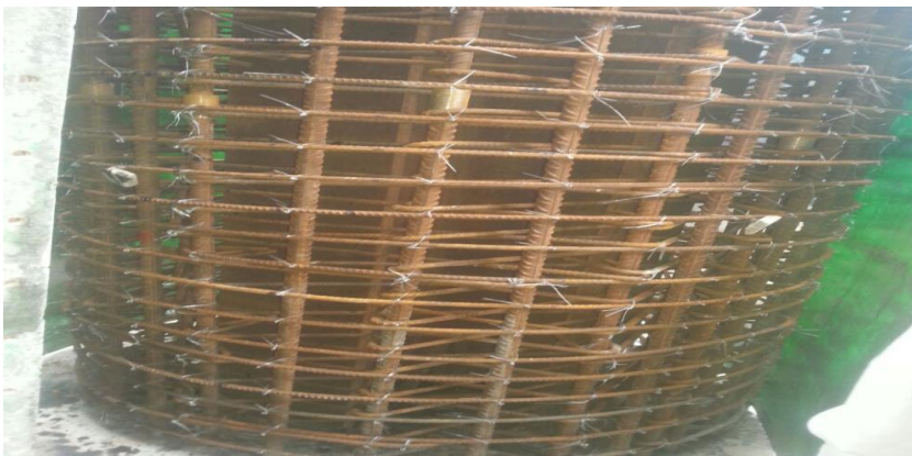
Figure 4.4: Mechanical Splice Reinforcement steel (photo from Commercial Bank of Ethiopia Head Office Building Construction)
