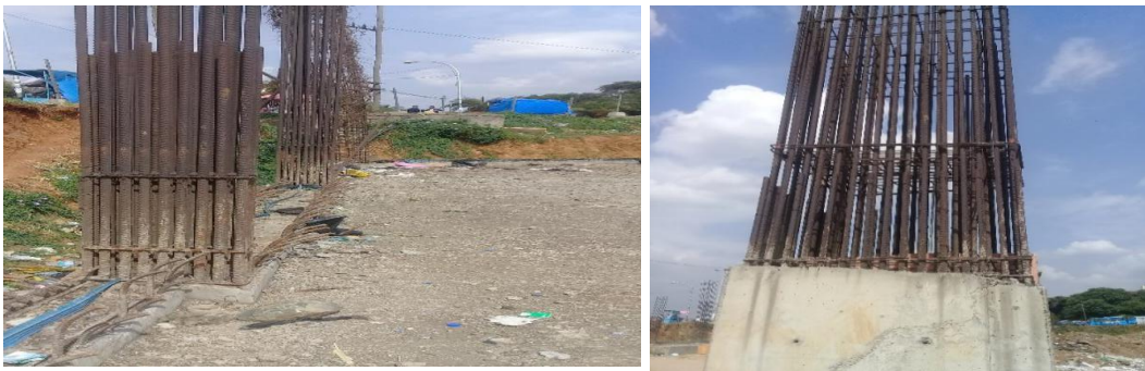
Figure 4.1: Reinforcement Steel Congestion Lap Splices (photo from Building Construction around Pissa in front of Adiss Abeba Municipality)
