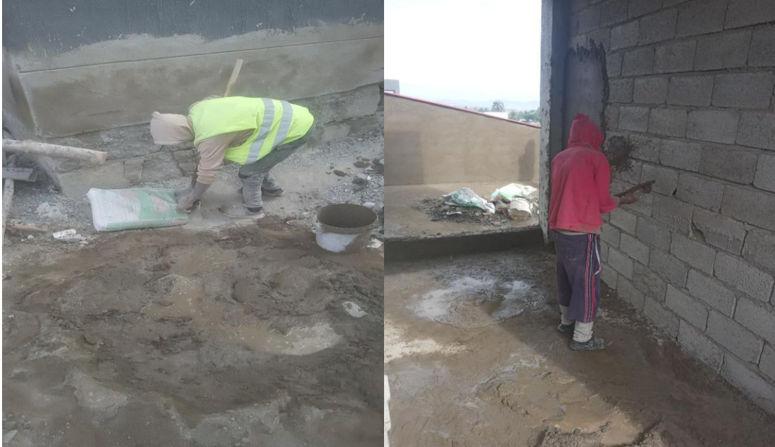
Figure 4-3: Plastering work covering above the dimension and improper way of work
