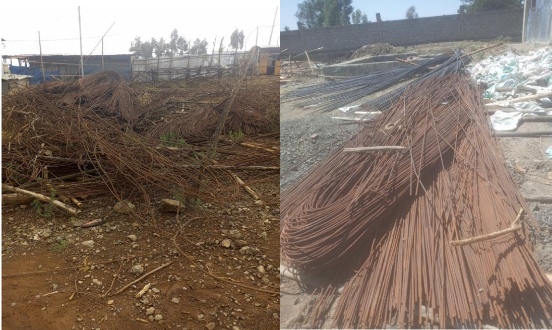
Figure 4-4: Improper put and unusable quantity of re-bar
