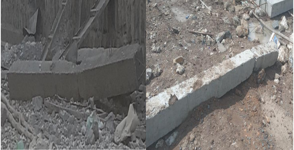
Figure 4-1: Damaged prefabricated concrete structure
