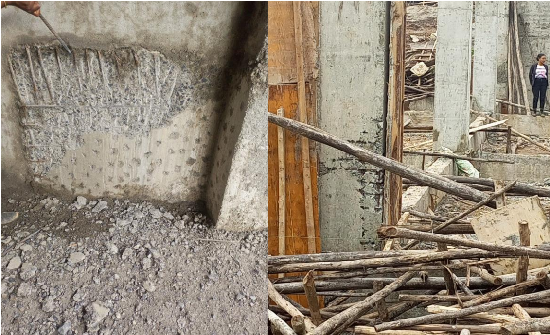
Figure 4-2: Bulged shear wall and segregated column structure in on-site construction site
