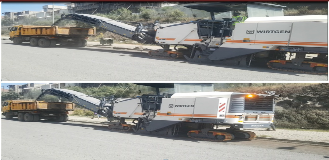
Figure 2.3: Milling machine removes asphalt pavement layer as part of pavement rehabilitation (photo at Yeshi Debele site).
