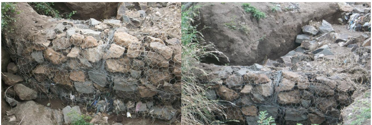
Figure 16: Use of Gabion for rehabilitation of degraded land within the study area
