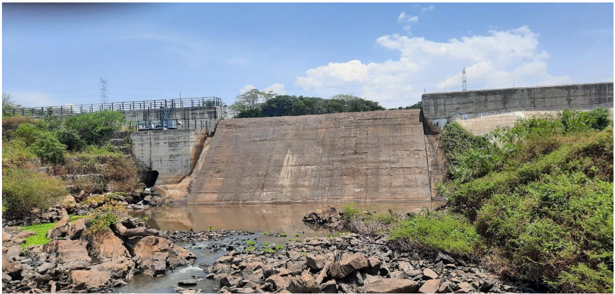
Figure 17. Environment flow gate and unregulated spillway for Kabalega reservoir (Photo 17 th /02/2020).
