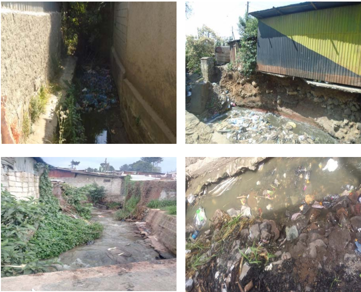
Figure 4.7: Flooding affected homes and disposal systems. (Source: Photos taken by the researcher).
