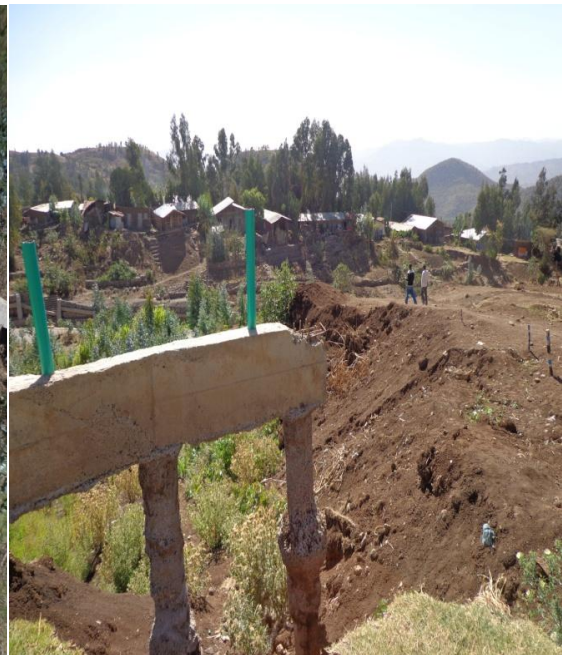
Plate 3.4 Sliding of Silty clay soil within constructed structure
