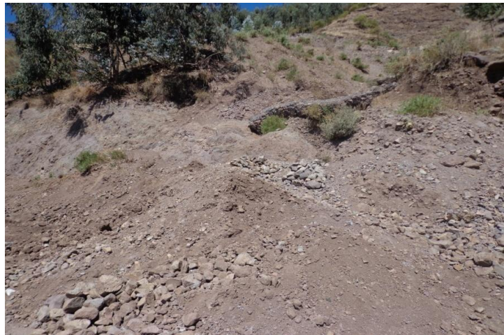
Plate 5.1 Due to lack of proper drainage slope material collapsed into road by rainfall in study area.
