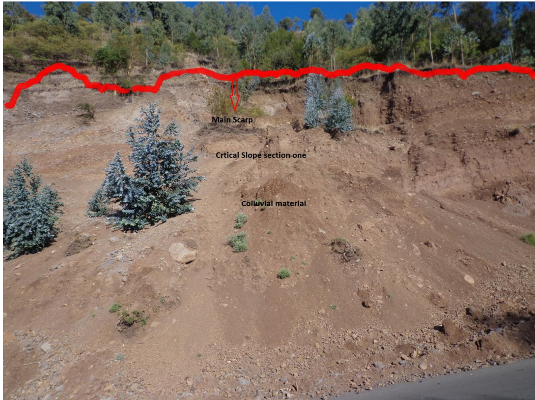
The movement of huge mass of colluvial material from steep slope to the side of the road
