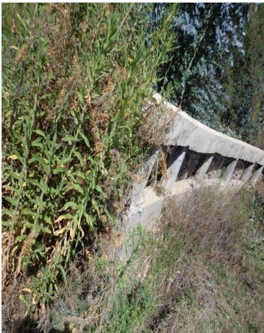
Plate 3.3 Displaced retaining wall near to school Building
