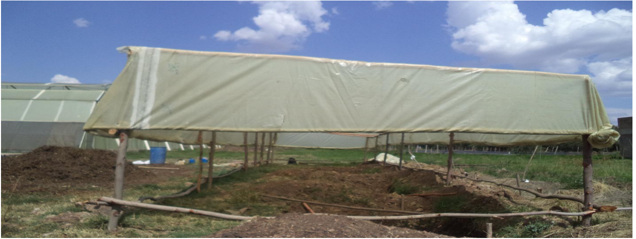
Fig.3. Treatment windrows and shed preparation at the beginning of composting in ZK
