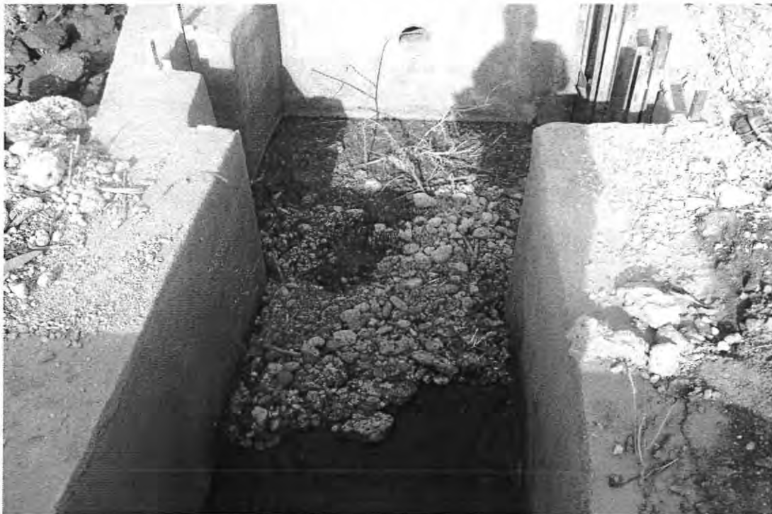
Figure 7: Shows Maintenance challenge of a canal (Picture taken from Gidara study site)
