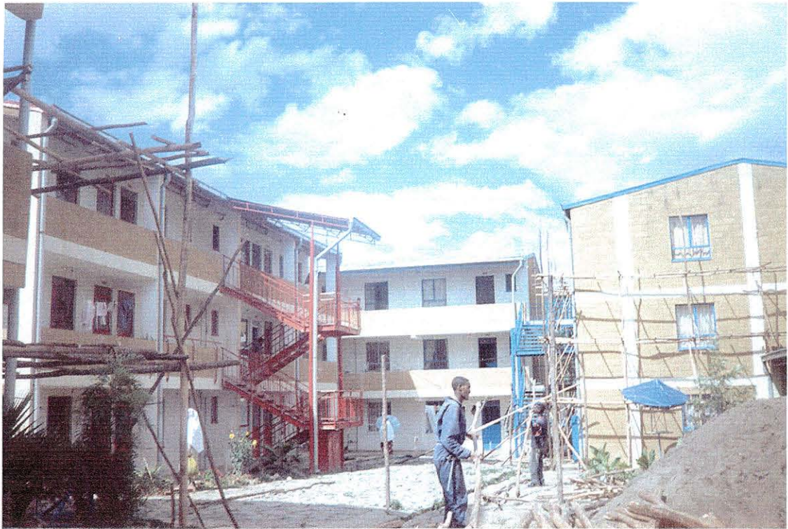
Figure 3.5: External wall plastering works in Kebena site. Photo taken from Kebena site.
