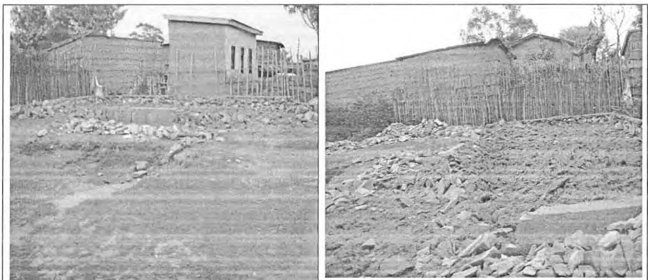
Picture 5.1 an Example of Bulldozed Houses in Tilte Kebele
