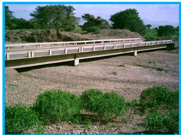
Photo 7: Baso River Bridge less than 0.7m clear opening height (Jun 2006)
