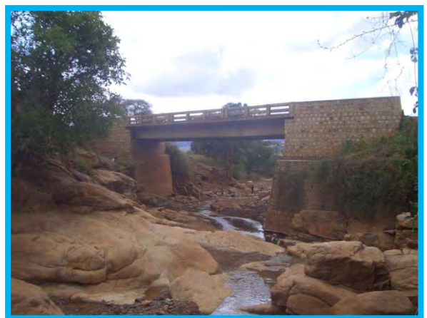
Photo 17: Degradation on river Warda exposing the foundation of the abutment (Aug 2007)
