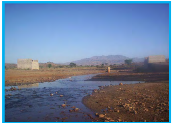
Photo 12: Failed Delbena Bridge (Aug 2006)
