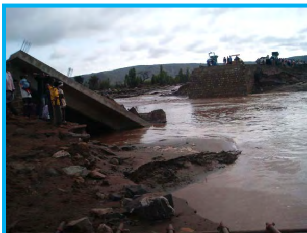
Photo 8: Failed Fafem River Bridge (Jul 2008)
