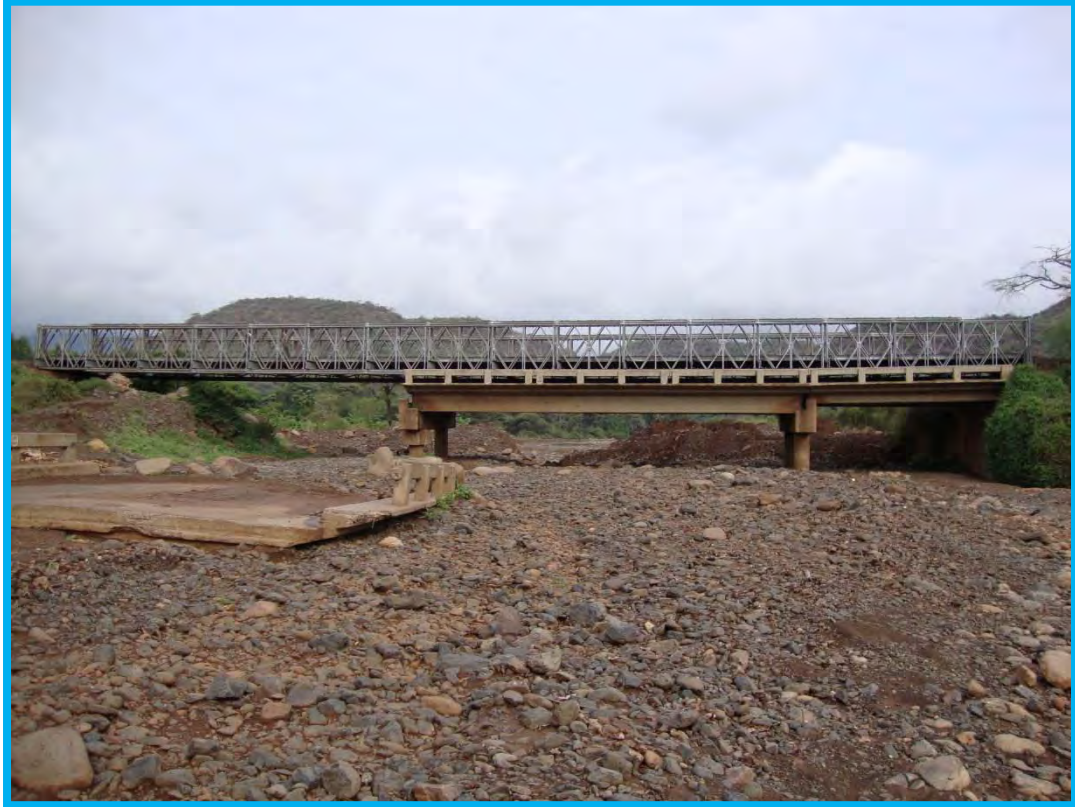
Photo 1: Raya River Bridge failure (Sep 2009)
