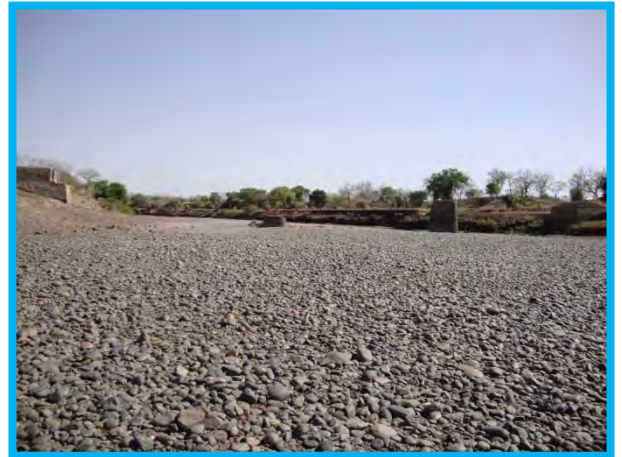
Photo 10: Failed Guang River Bridge (Jun 2009)
