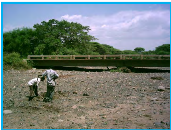
Photo 6: Shefe River Bridge less than 0.9m clear opening height (Jun 2006)
