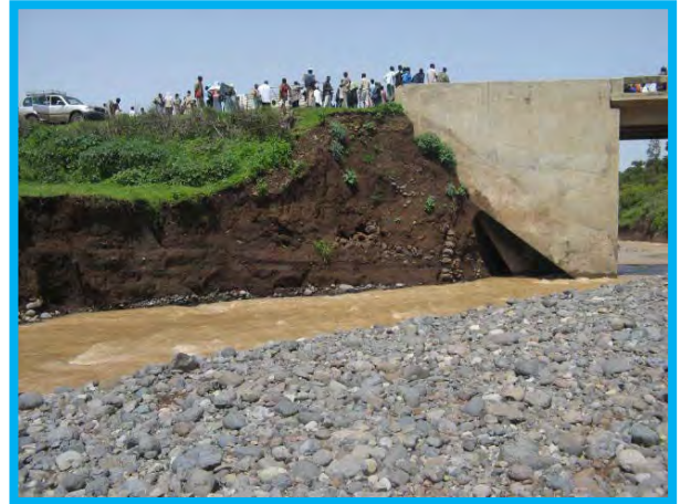
Photo 15: Scouring on the abutment of Garno Bridge (Jul 2006)
