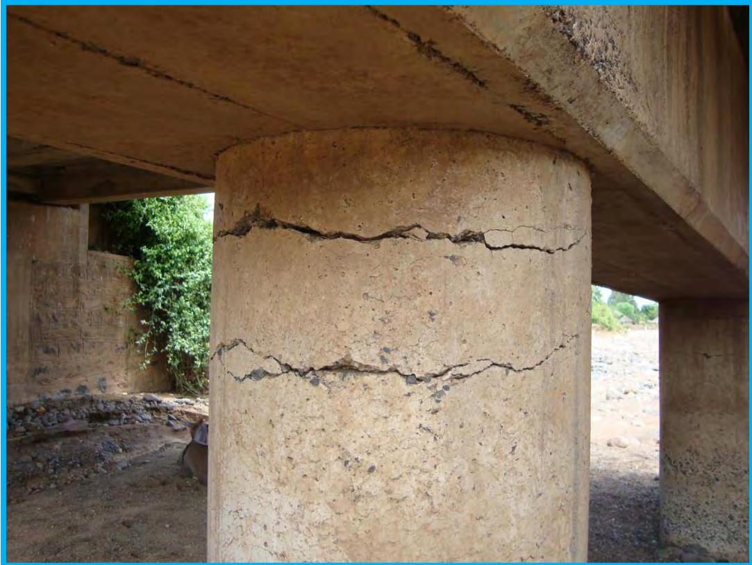
Photo 2: cracks on the pier (Sep 2009)
