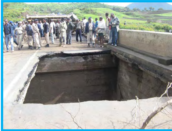
Photo 14: Collapsed approach slab of Garno Bridge (Jul 2006)
