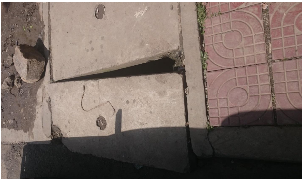
C. Manhole cover misplaced and partly closed the opening
