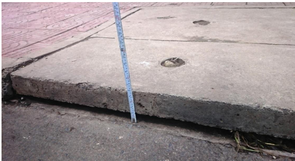
A.Manhole opening depth less than 5 cm
