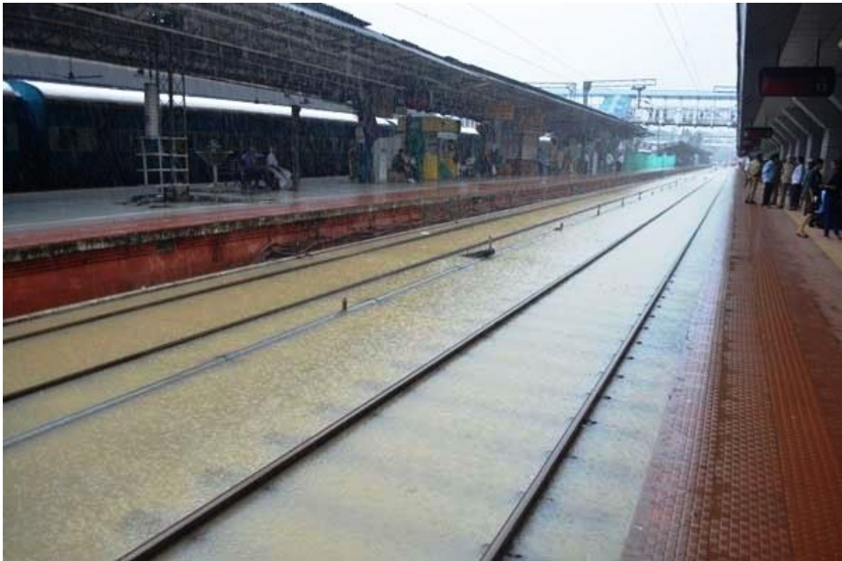
Figure 2.4: Railway track flooding (Thiruvananthapuram, India)
