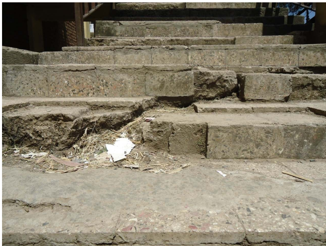
Figure 1. Example of the cracked & broken up and down stairs of seba dereja from the Piasa main road along to the ENADB.
