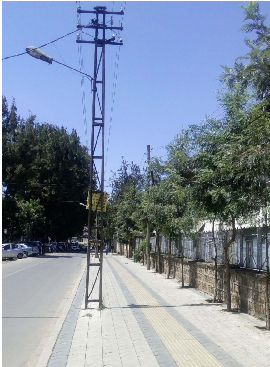
Figure 5. Example of electric pole around the entrance of ENADB
