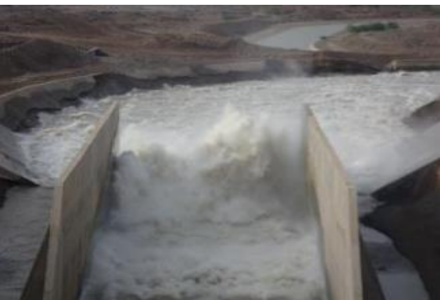
5: Flow after Stilling Basin
