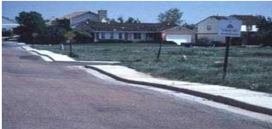
Figure. 2.7 A View of Road Undergoing Volume Change
