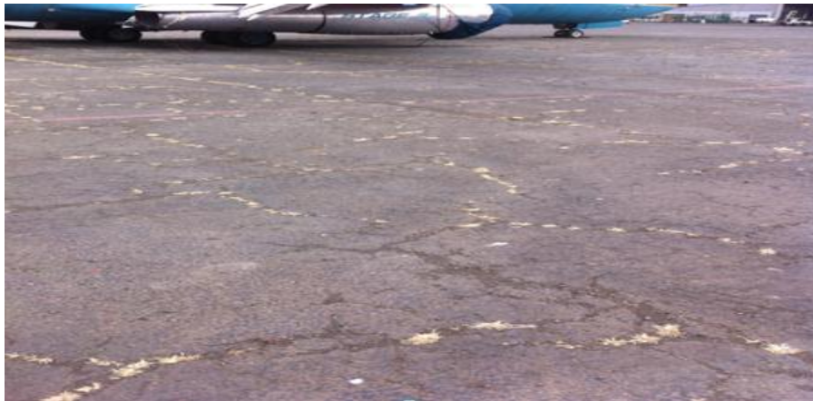
Figure 1.2 Exiting Apron Crack at Bole Site
