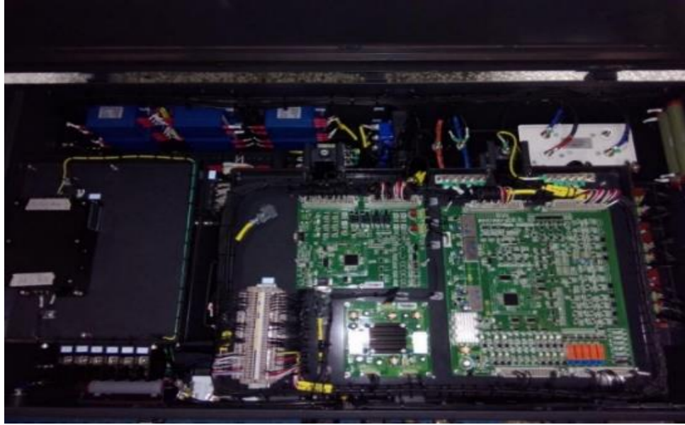
FIGURE 11: SHOWS THE AUXILIARY POWER SUPPLY SYSTEM AT AALRT
