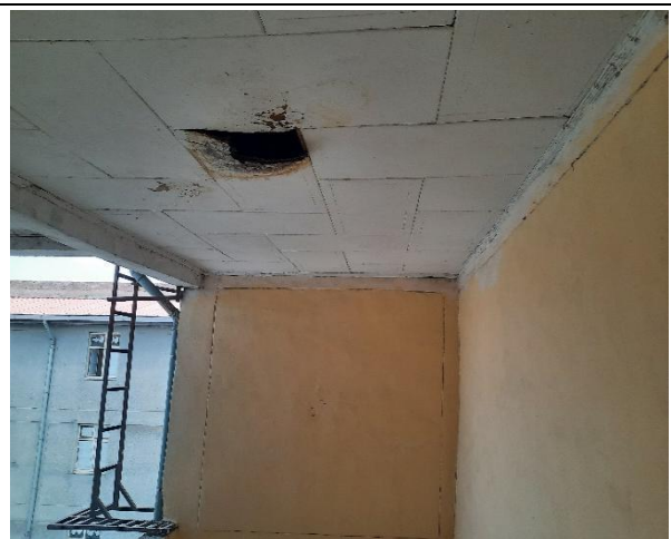
Figure 4.4 photos showing defects due to leakages
