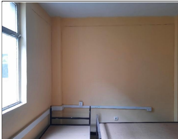
Figure 4. 3: Photo showing external electrical installation
