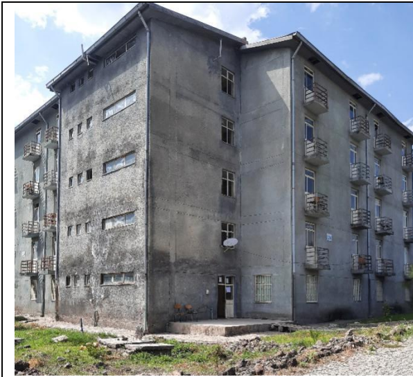
Figure 4.5: Photo showing defects on the external facade
