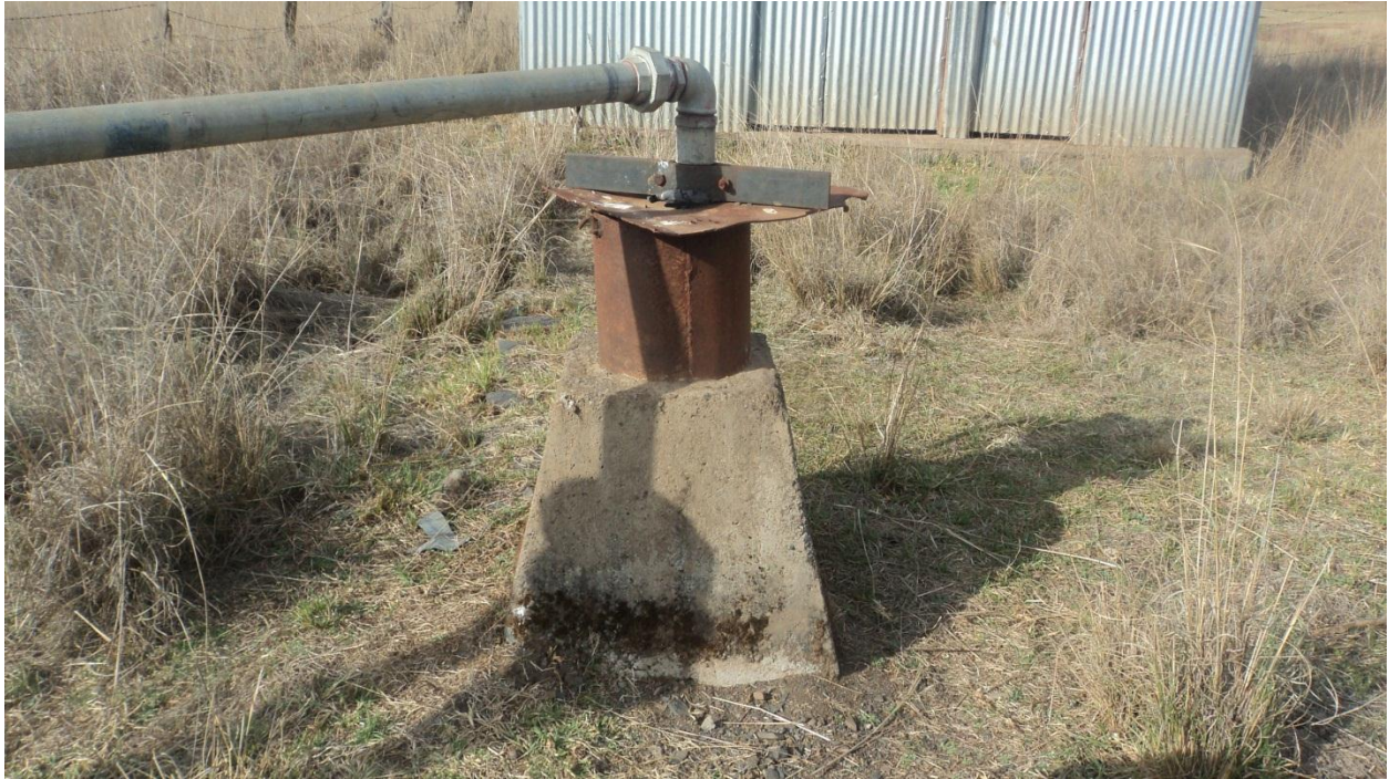
Figure 7-6 Gaba jimata water supply deep ground water fitted with submersible pump
