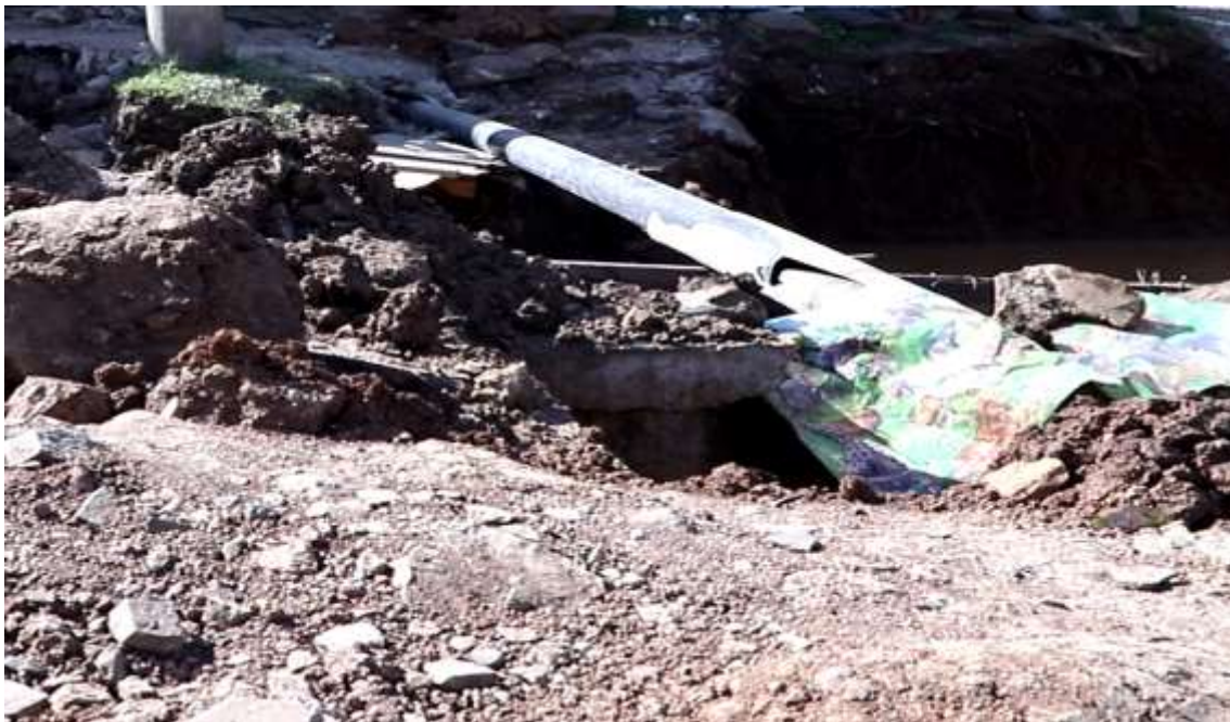
Figure 1.1: Inaccessible pedestrian road around workplace, with construction materials blocking the path.
