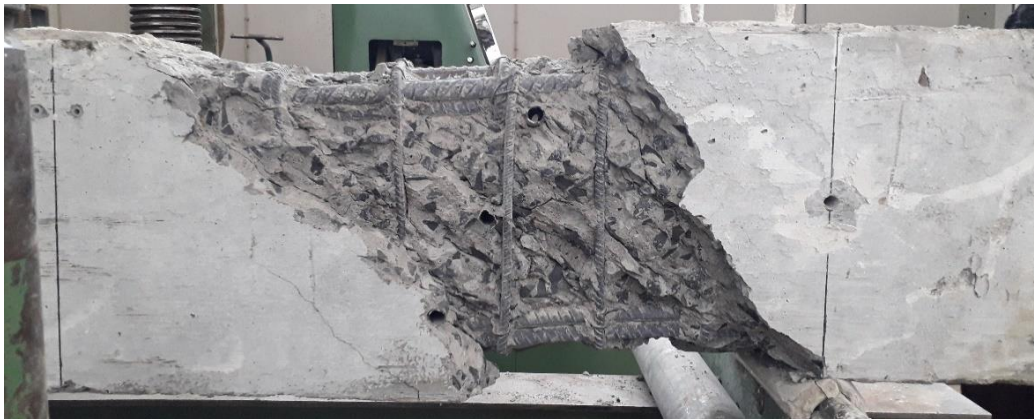
Figure 6-28: Spalling on Both Sides of the Beam
