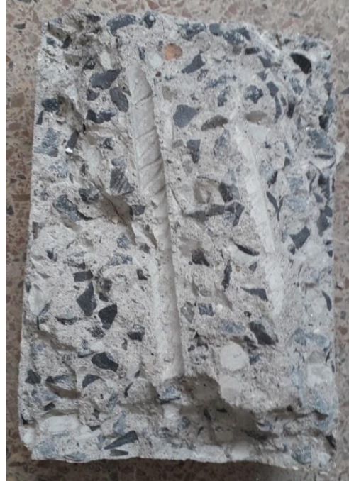
Figure 4-38: Spalled off Section (SIII8-75)
