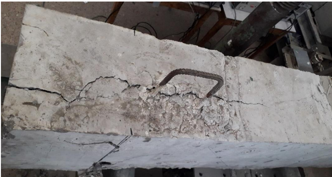
Figure 4-31: Top Longitudinal Crack (SIII10-75)
