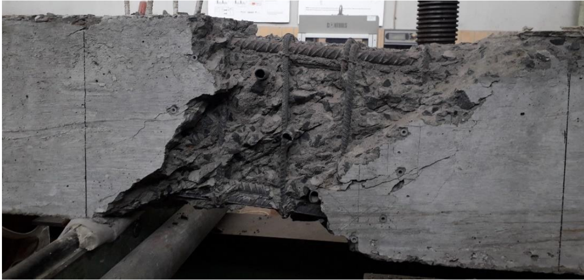
Figure 4-26: Spalled Section Back Side (SIII10-50)
