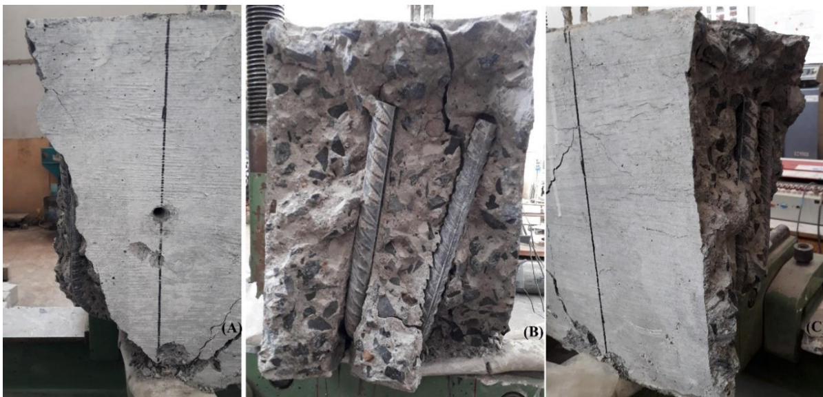
Figure 4-37: Concrete Cover Spalling at the Rear Left End (A) Front View (B) Sectional View (C) Back View (SIII8-75)
