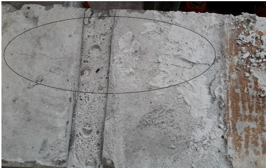
Figure 4-45: Top Longitudinal Crack (SIII0-75)
