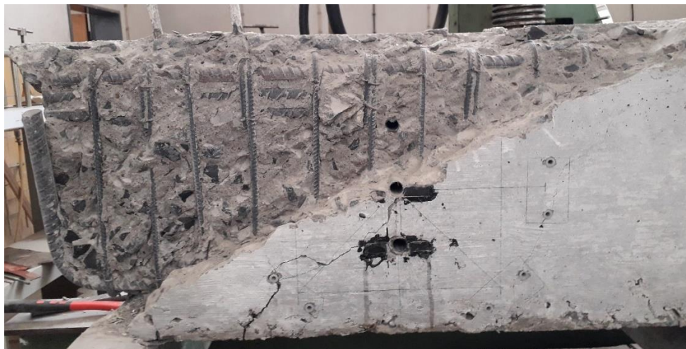
Figure 4-41: Spalled Section Front Side (SIII8-75)
