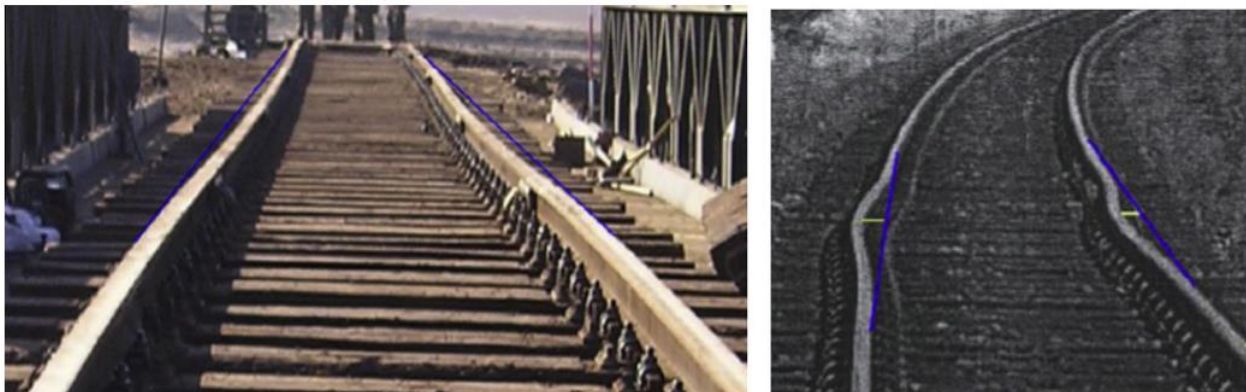
Figure 1. 1 Visual appearance of a deteriorated ballasted railway track [9]
